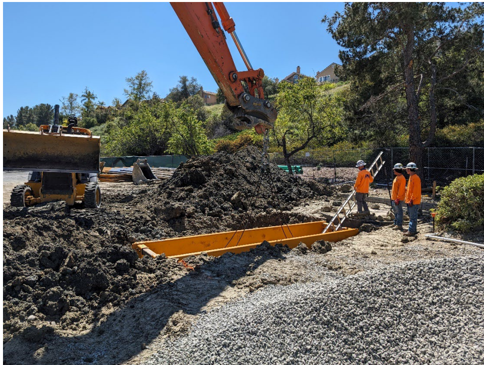
PHC started to excavate and support trench for 12-inch PVC Gravity Pipeline.
