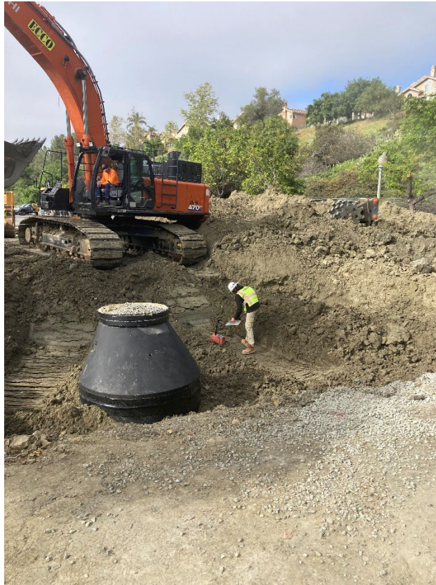
GMU Soil Technician field observing and assessing backfill and compaction efforts by nuclear gauge.
