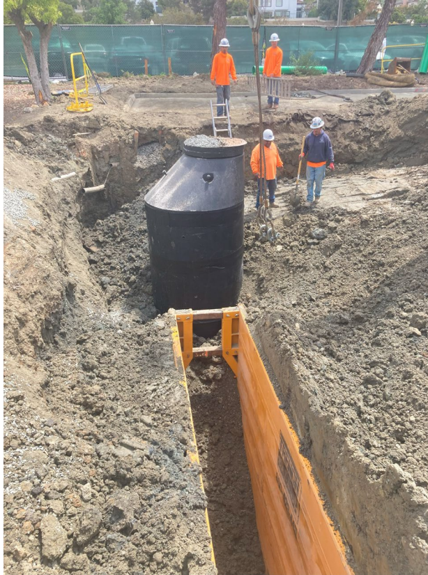
Backfilled and compacted materials for 12-inch PVC Gravity Pipeline and Diversion Manhole.
