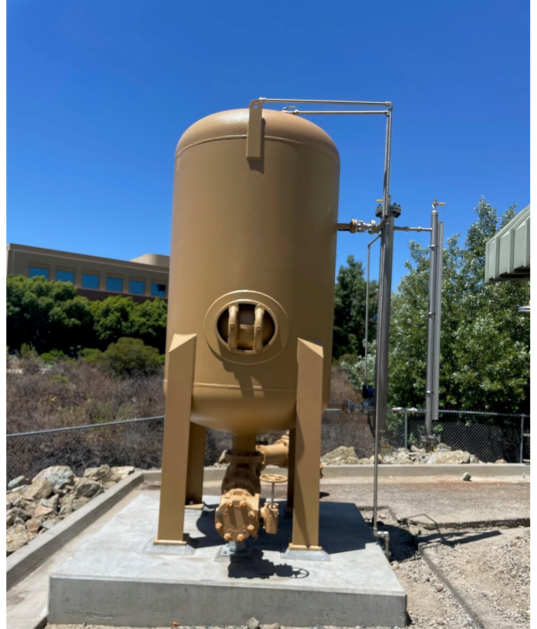
New 1,100 Gallon Surge Tank
