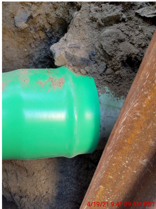
New 8-inch Sewer Line and Point of Connection to Existing Sewer Line
